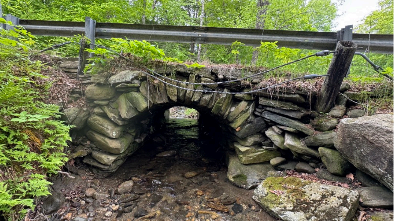
Downstream end. Note the stones on the south side (left) at the bottom of the arch appear to be sloped downward, but are in fact well supported and secure. The spandrel and wing walls are in very poor condition and need rebuilding.
