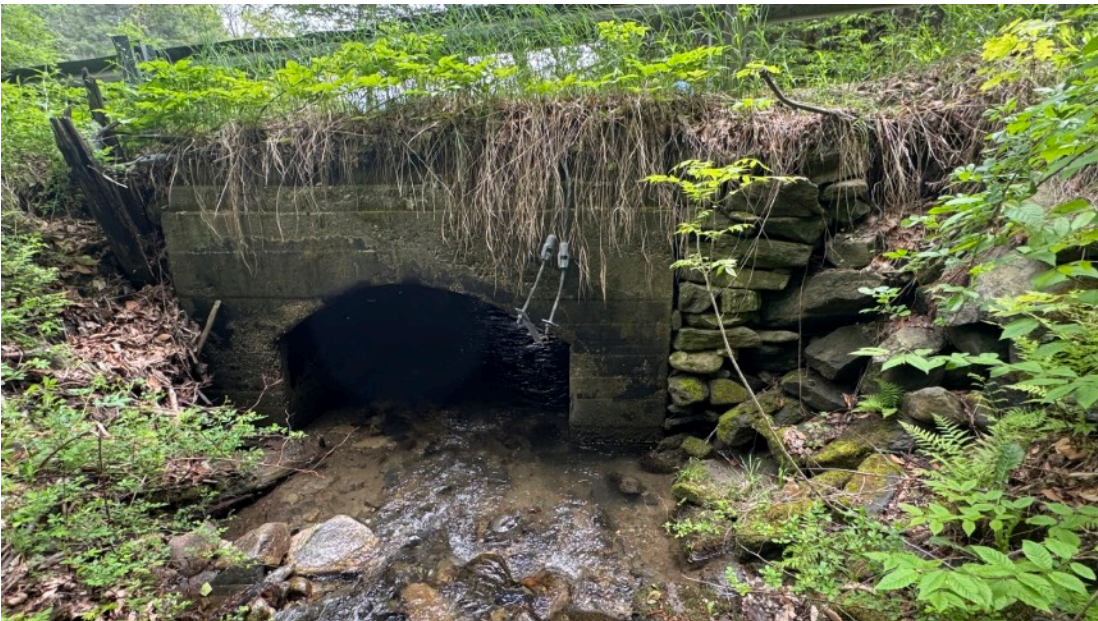
Upstream end. Concrete is stable but the stone wing walls are deteriorating, particularly the one to the south (right).
