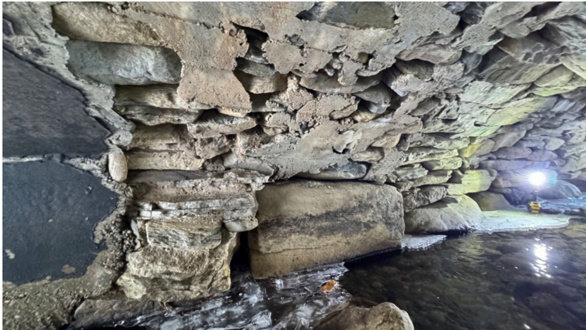
North side of middle section. Shows poor building technique, but it appears to be relatively stable
