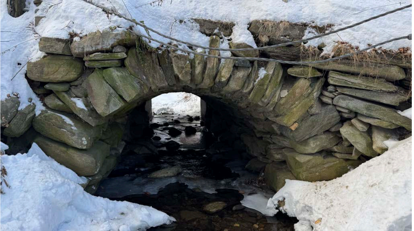
Downstream end. Note the stones on the south side (left) at the bottom of the arch appear to be sloped downward. This may indicate a problem with this section. Both wing walls are in poor condition.
