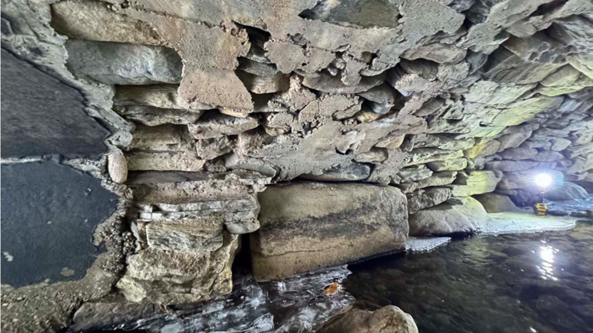
North side of middle section. Shows poor building technique, but it appears to be relatively stable
