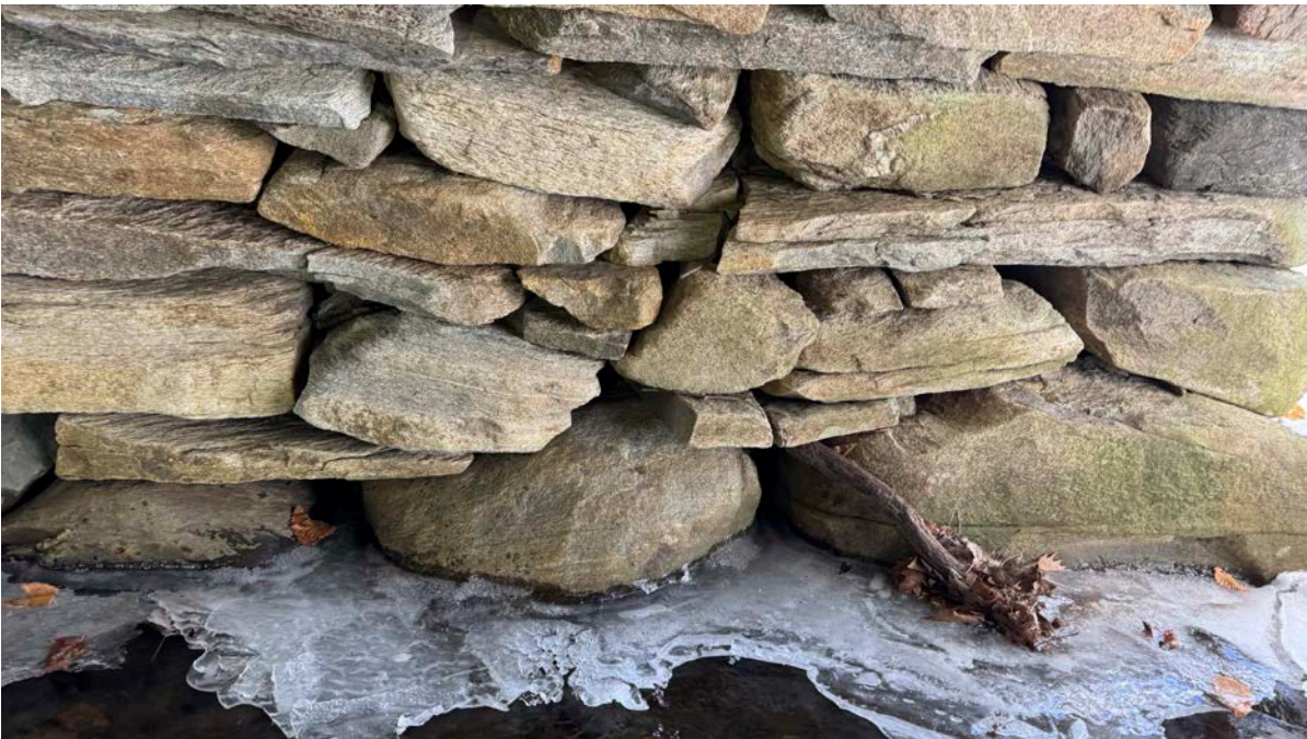
North side, downstream portion, shows some cracked stone and mortar loss, but is generally in good condition.
