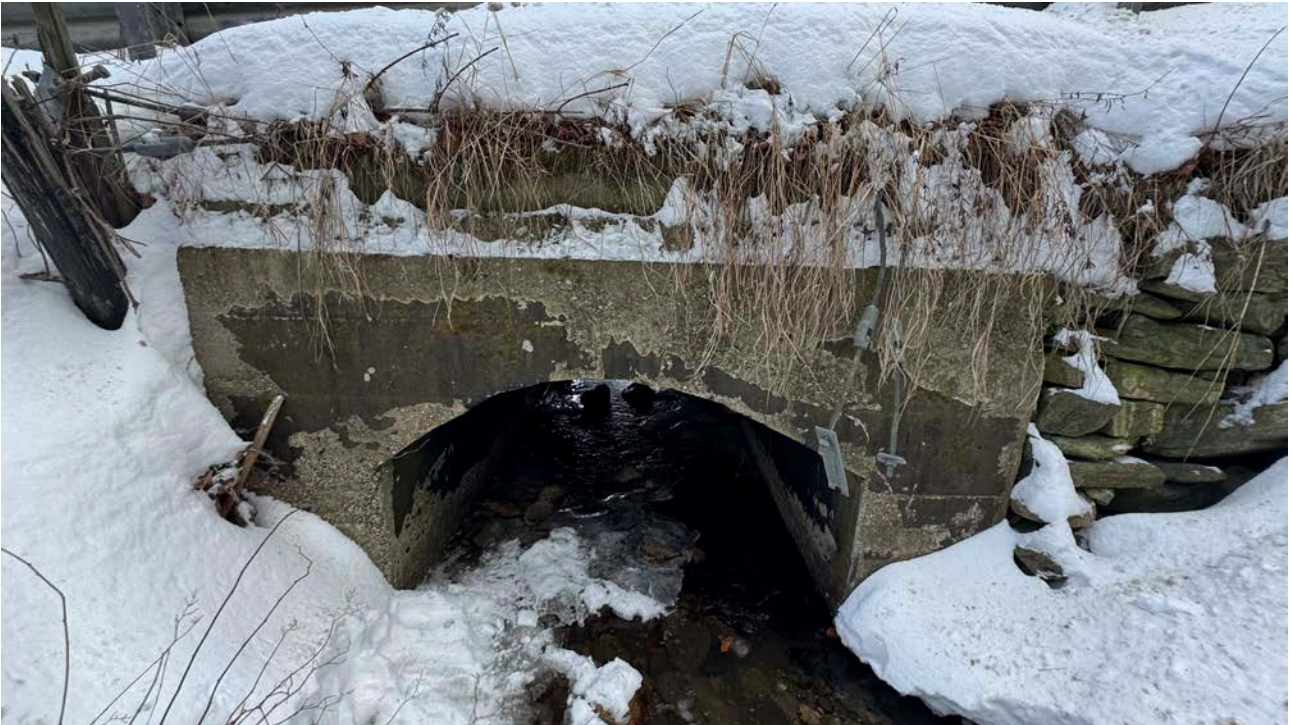
Upstream end. Concrete seems stable but the stone wing walls are deteriorating.
